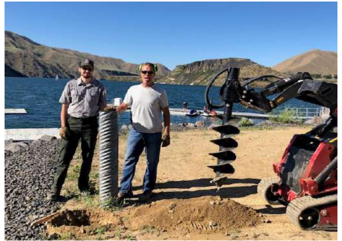
A big thanks to the U.S. Army Corps of Engineers Colin Byers and Dan Smith for drilling holes and setting sleeves for the three masts plus help from Lauren Howard for leveling our Headquarters with concrete blocks.
