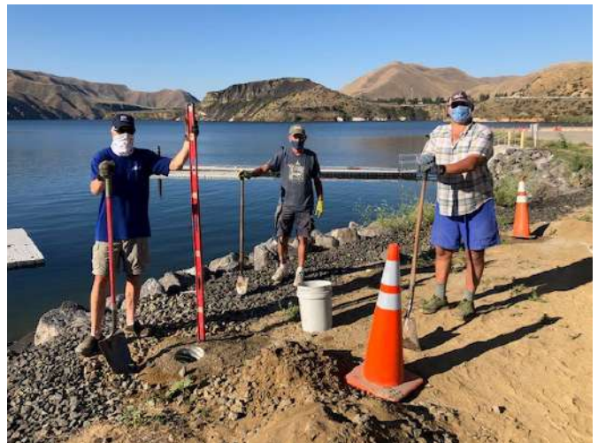
Steve Christiansen, John Gabiola and JT More finishing up the footings Twenty-two bags of Sakrete in the ground.
