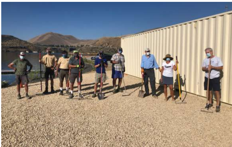
Morning Gravel Workshop: Thanks to our many volunteers and Idaho Dept. of State Parks and Recreation - 13 cubic yards in place in one hour. Thank you Rushmann Sand and Gravel for the gravel.
